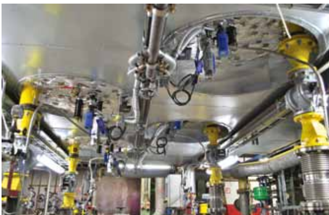
Typical DDZG system, here with upshot burners
