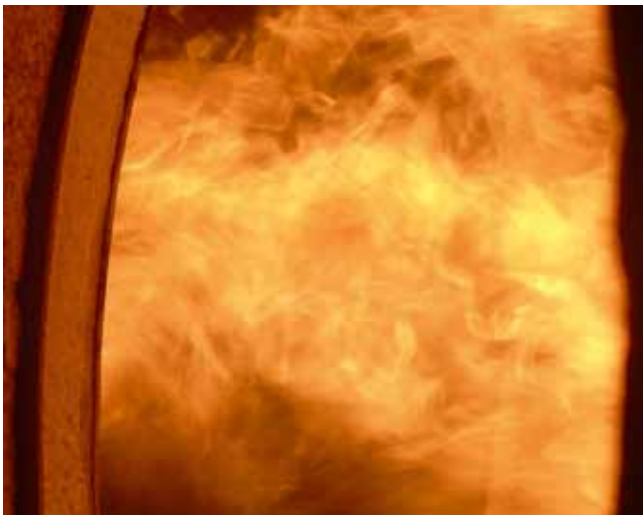
Typical DDZ-M heavy fuel oil flame
