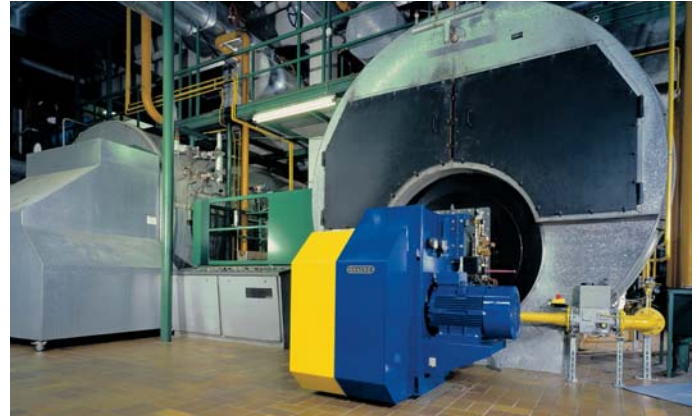
The photograph shows a plant with a TEMINOX® GLS 95-22 monoblock burner on a 13.2 t/h three-pass boiler.
