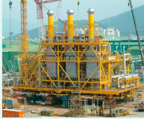
Boiler Set for Dalia FPSO
